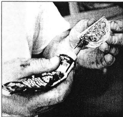
A heat riser block-off plate had to be manufactured. A little more Permatex black silicone helps seal the deal.
